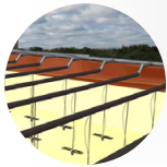
Air piping floats on water surface
